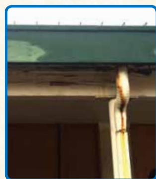
Leaky roofs are in need of replacement.
